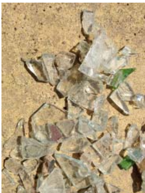
Glass picked up from the surface at Coaley after the topping was added
